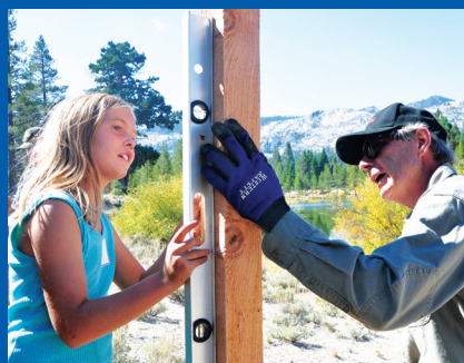
Volunteers of all ages came together for this year's Tahoe Forest Stewardship Day. New fence posts were installed as one of the stewardship activities at Tahoe Paradise Park in Meyers, CA.
