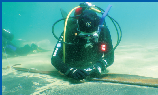
Divers work to secure bottom barriers with steel rebar as part of an effort to control invasive species in Lake Tahoe. A new control effort was launched in late October to control Asian clams at the mouth of Emerald Bay. (Photo courtesy Tahoe Resource Conservation District.)
